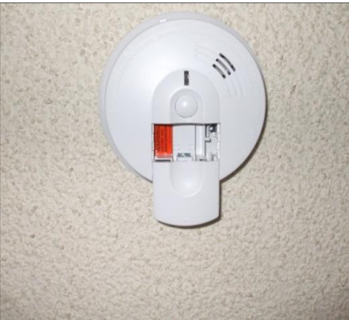
Non-functioning smoke detector
