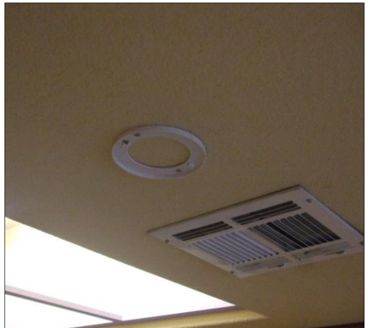
No smoke detector
