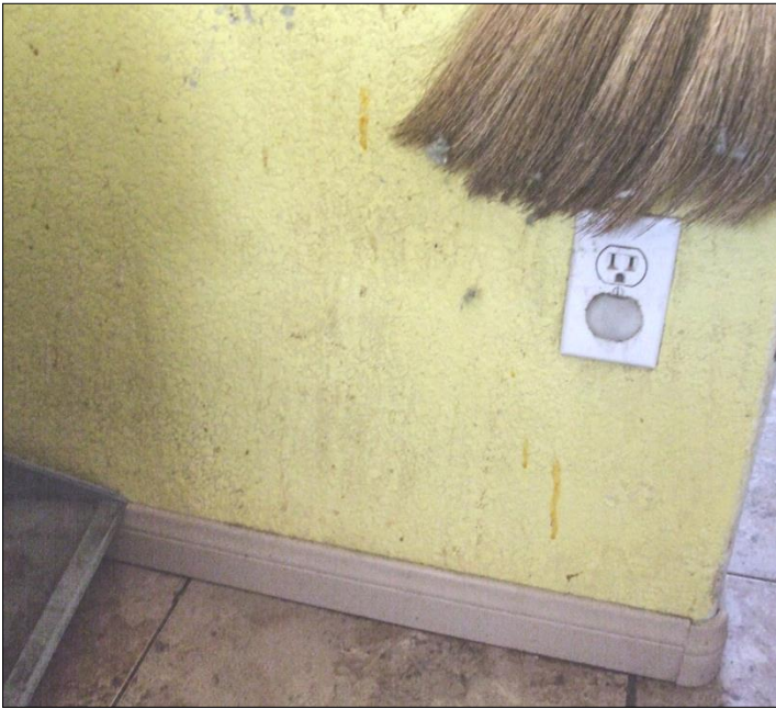
Dirty kitchen wall
