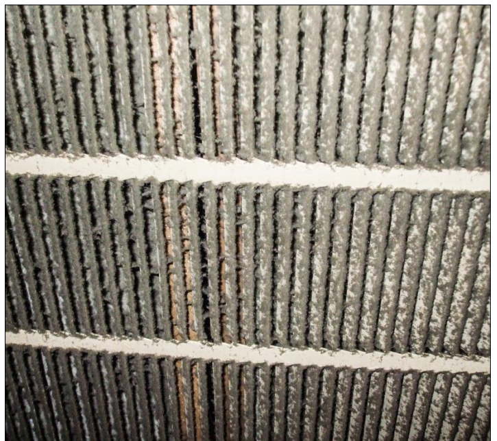
Dirty air filter and vent
