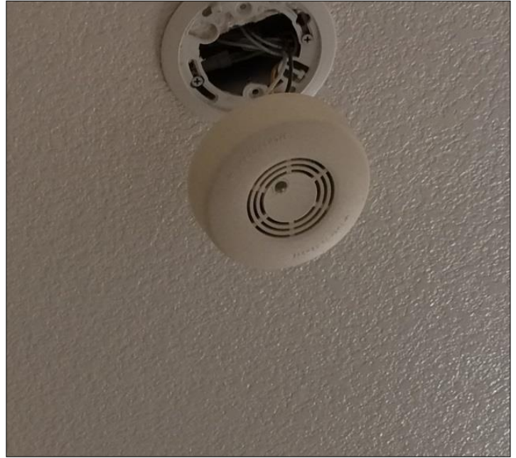
Non-functioning smoke detector
