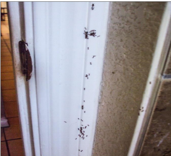
Insects from bathroom floor up wall to top of door frame
