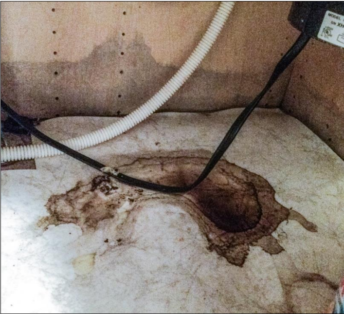
Water damage and mold
