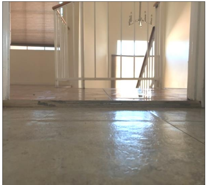
Tripping hazard – uneven flooring leading downstairs
