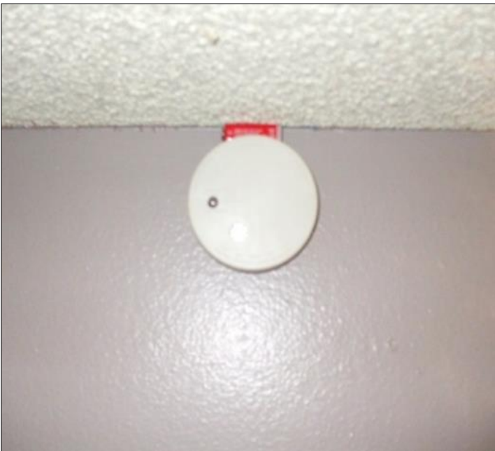
Non-functioning smoke detector with battery on top
