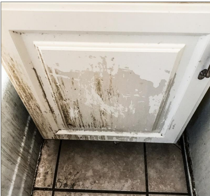
Filth and mold on bathroom floor, tub, and cabinet
