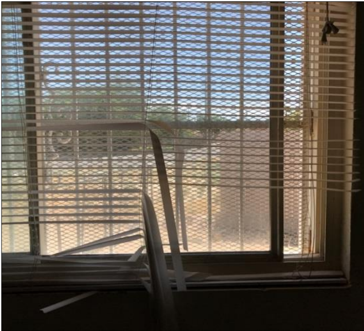
Broken and dirty bedroom window blinds
