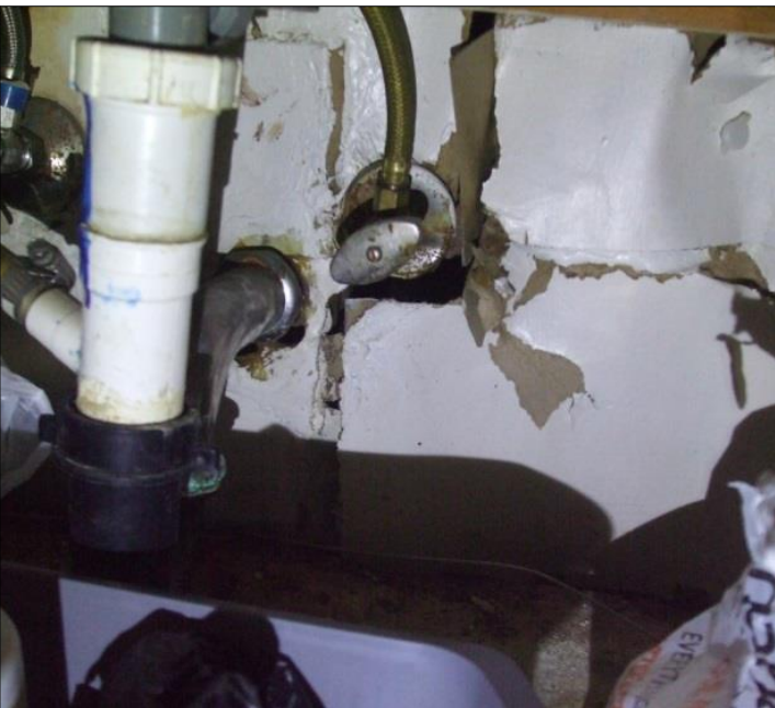
Wall damage under sink
