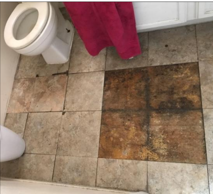
Water damaged 2nd floor bathroom
