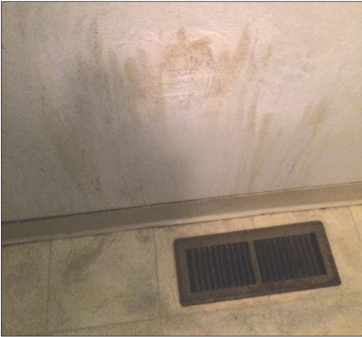
Dirty bathroom walls
