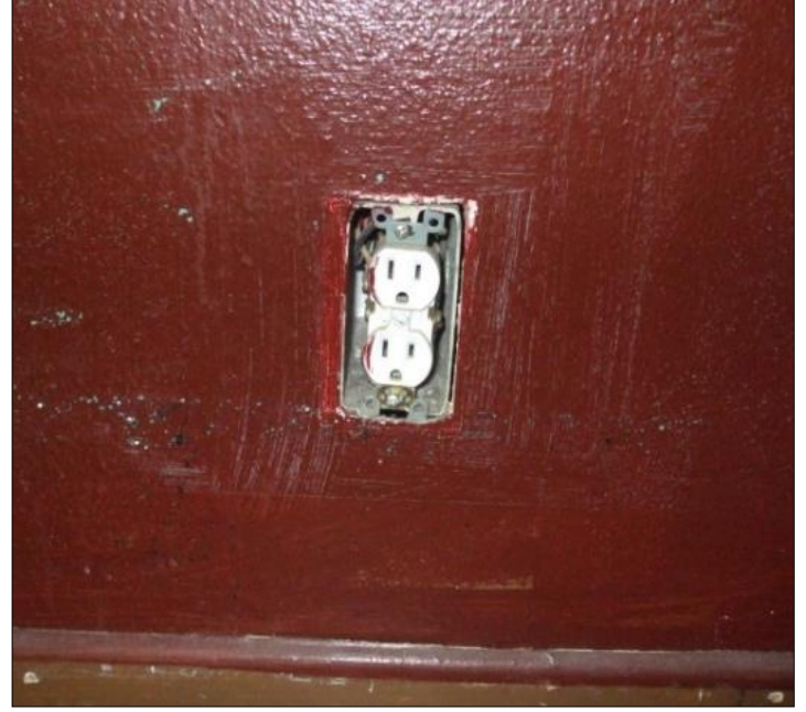
Exposed electrical outlet
