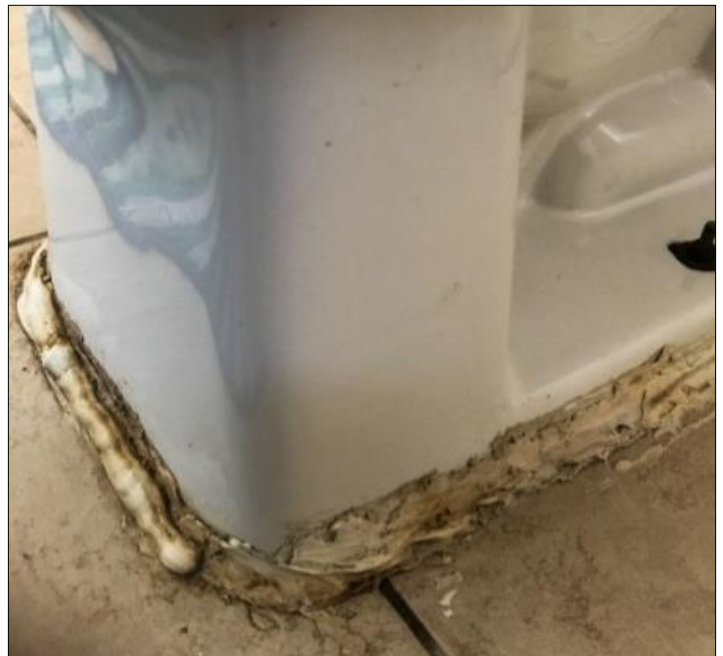
Leaking, moldy toilet
