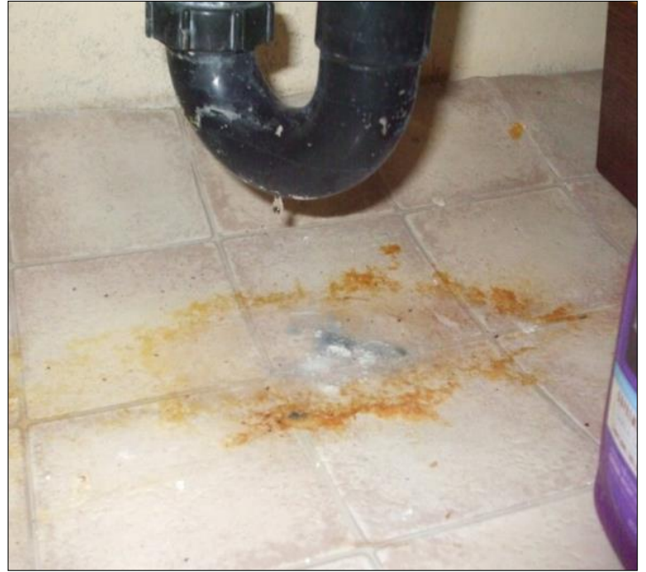
Water damage and mold under sink
