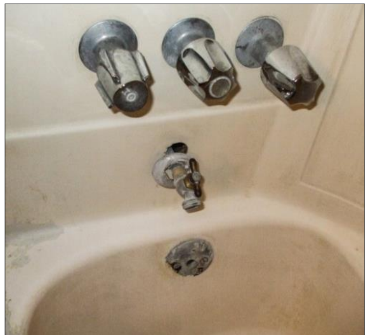
Dirty bathtub with broken water spigot
