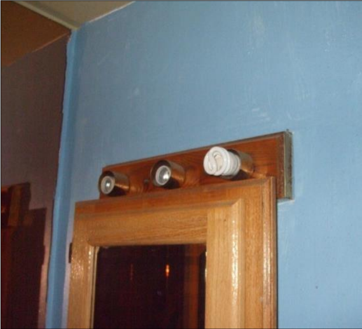
Bathroom light missing lightbulbs and not functioning Home 20
