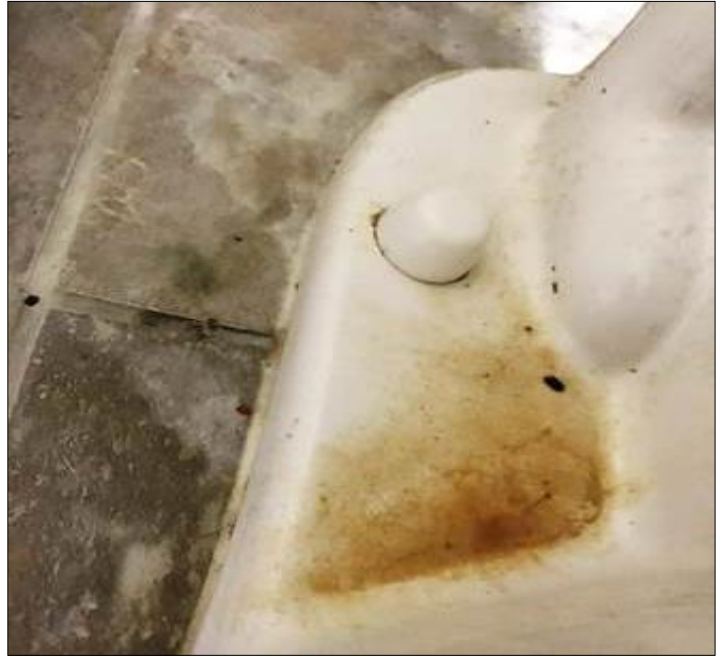
Dirty and leaking toilet
