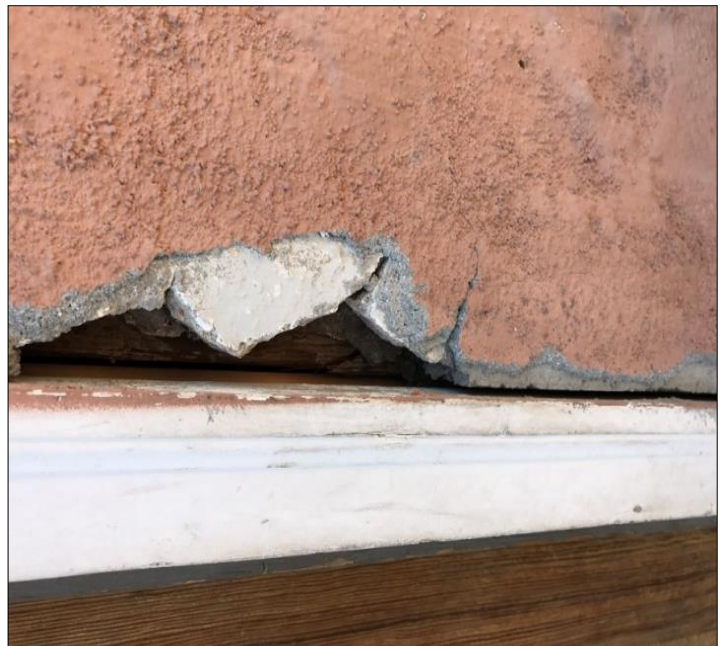
Exterior wall damage above door
