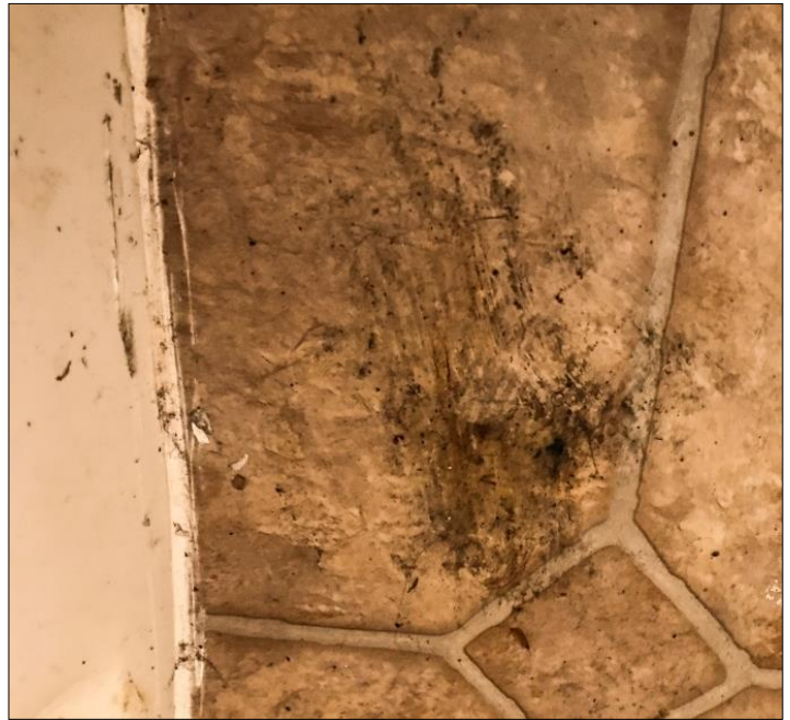
Feces on bathroom floor
