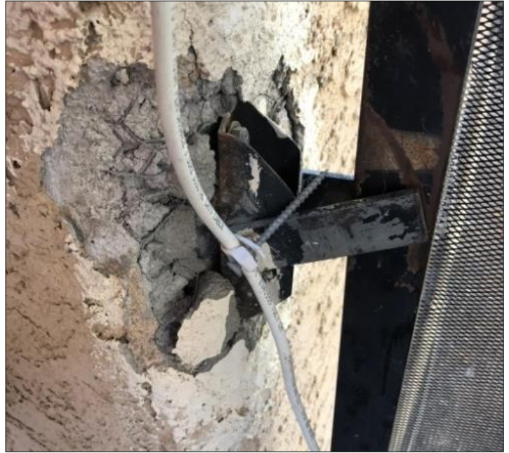
Exterior wall damage
