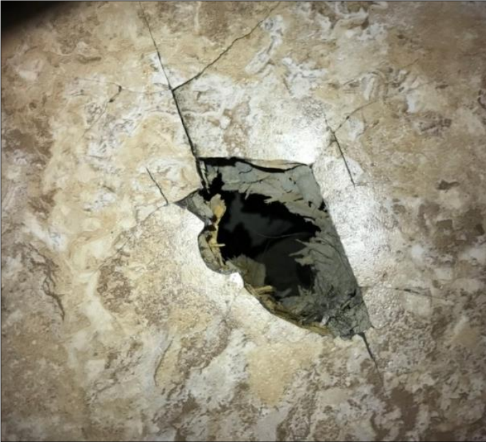
Approximately 4" x 8" hole in 2nd floor bedroom between two beds
