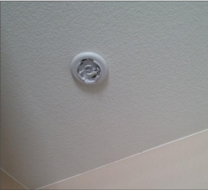
No smoke detector
