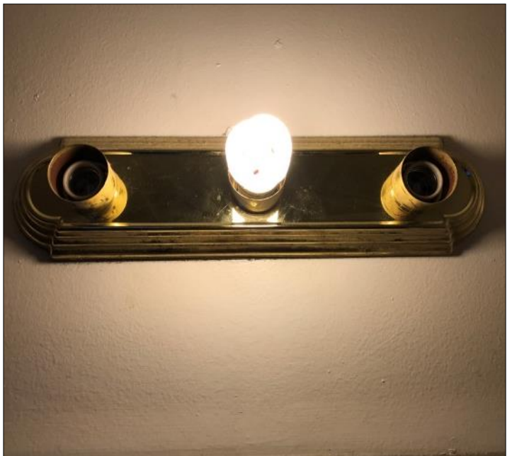
Only one lightbulb for bathroom and bedroom; client indicated no response to complaints Home 35
