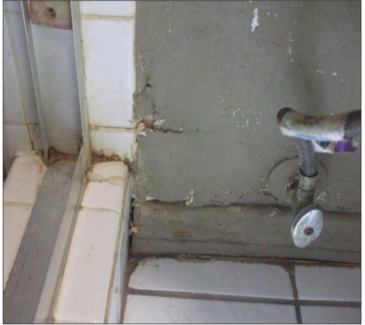
Water damage and mold
