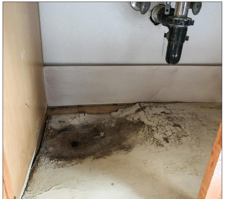
Bathroom sink water damage
