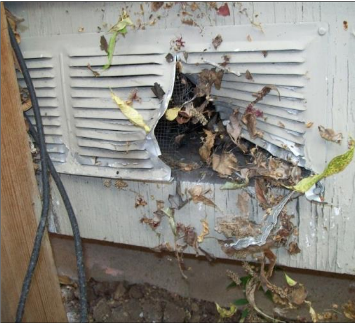
Exterior vent damage
