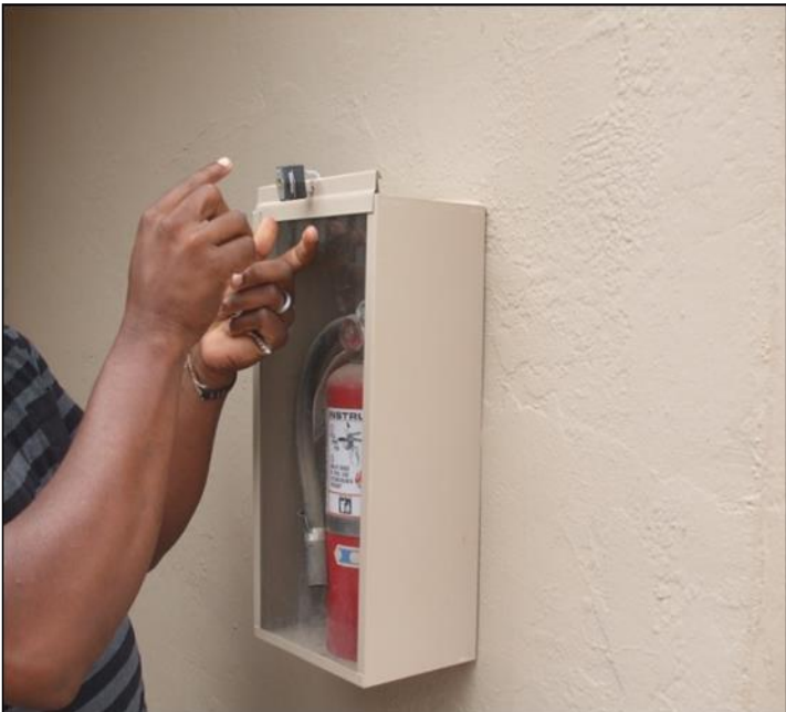
Caregiver trying to find key to inaccessible, old fire extinguisher
